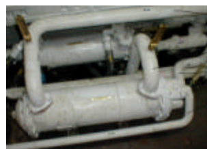
FIGURE. 10 FRESH WATER MAIN COOLER ON THE SHIP “NASE MORE”
