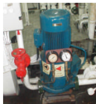
FIGURE. 8 SEA WATER PUMP ON THE SHIP “NASE MORE”
