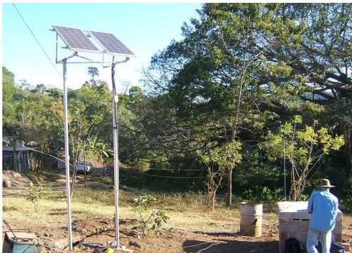
FIGURE 5 EL SALVADOR PHOTOVOLTAIC SYSTEM
