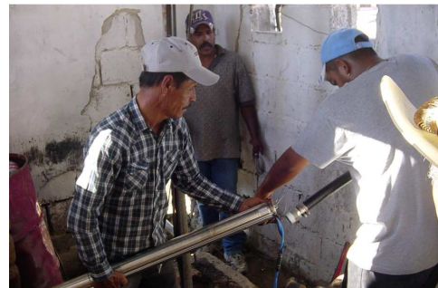
FIGURE 3 MEXICO: INSTALLATION OF SOLAR WATER PUMP
